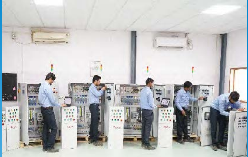
Industrial Automation: Control Panel Building
